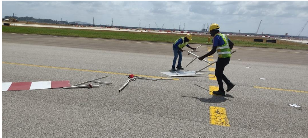
Figure 5: The damaged marker board
