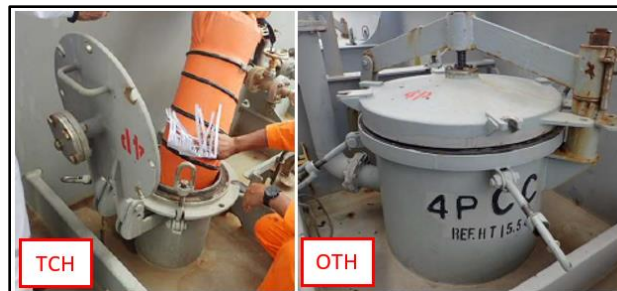
Figure 4b – Portable air chute connected the TCH and OTH cracked open ( Source: the Company )
