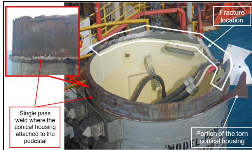
Figure 9a – View of the single pass weld and fracture location at incident crane pedestal ( Source: the Company )
