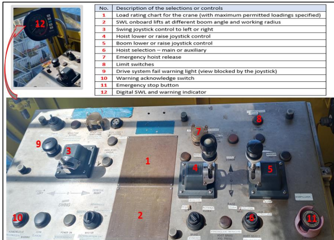
Figure 5 – Layout of the control panel (inside the no.2 crane cabin) (Source: the Company)
