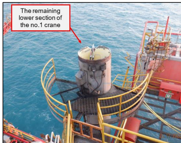
Figure 1 – View of the remaining lower section of the no.1 crane (Source: the Company)
