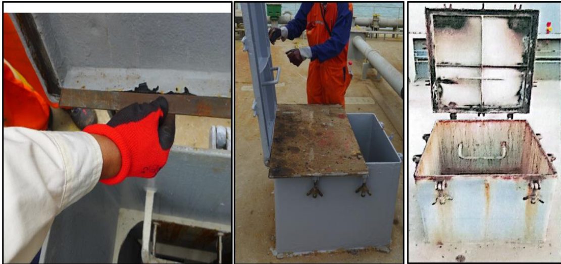
Figure 5: The picture on the left shows an example of the replacement metal piece to be welded at the lip. The centre picture shows the wet wooden plank covering the opening. The picture on the right shows the completed welding by the FT on the booby hatch, aft of CH3.
