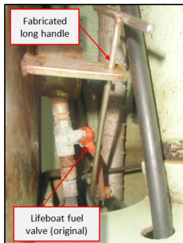
Figure 6 – View of the long metal rod fabricated for ease of opening/closing the fuel valve (Source: the Company)
