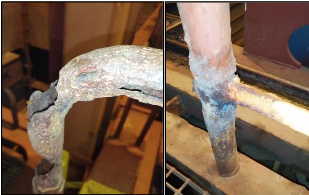
Figure 4: Some of the corroded and holed railings found along the catwalks and cross decks
