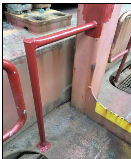
Figure 6: New installation of railing at cargo hold no.3 (Source: ZEABORN SHIP MANAGEMENT GMBH & CIE. KG)
