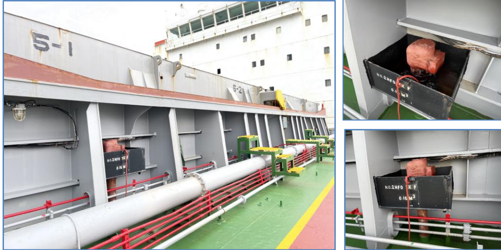
Figure 3 – View of the forward vent for No.2 HFO tank (Port) - (Source: The Company)
